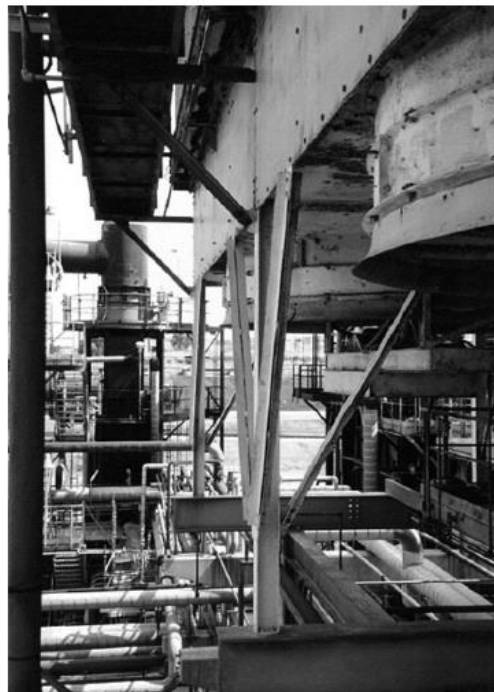
FIGURE C13.6-1 Fin Fan Elevated on Integral Supports
