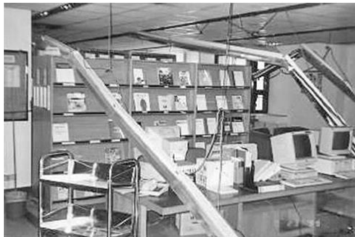
FIGURE C13.1-3 Collapsed Light Fixtures
