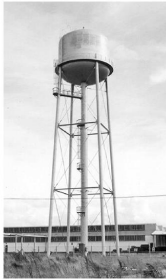
FIGURE C15.1-1 Steel multilegged water tower
