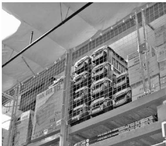
FIGURE C15.5-1 Merchandise restrained by netting
