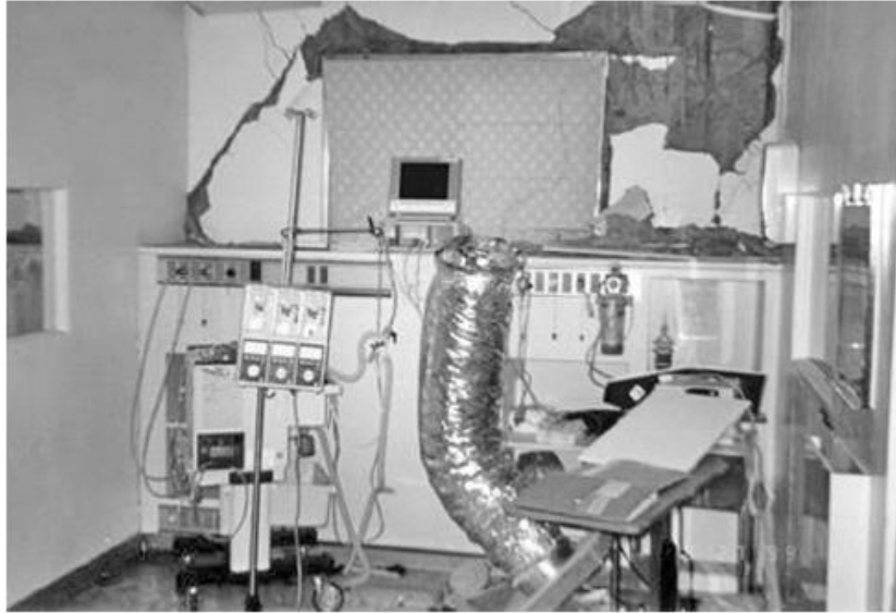
FIGURE C13.1-6 Collapsed Duct and HVAC Diffuser
