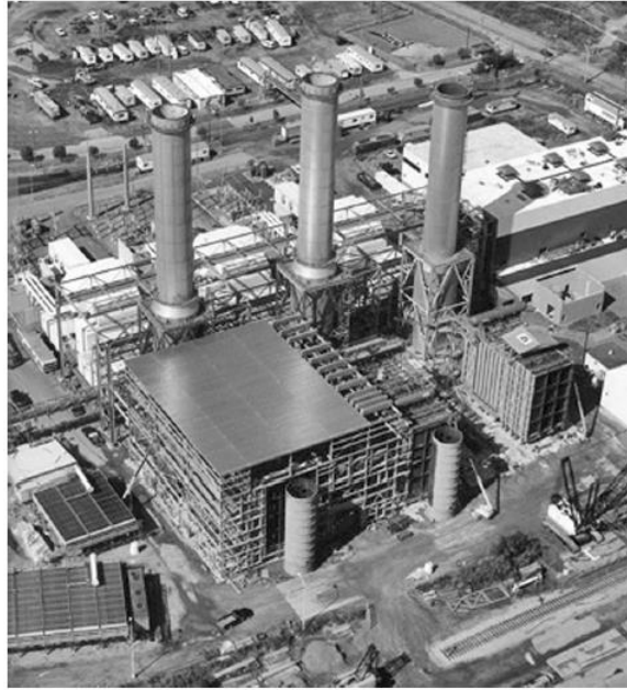
FIGURE C15.1-3 Heat recovery steam generators
