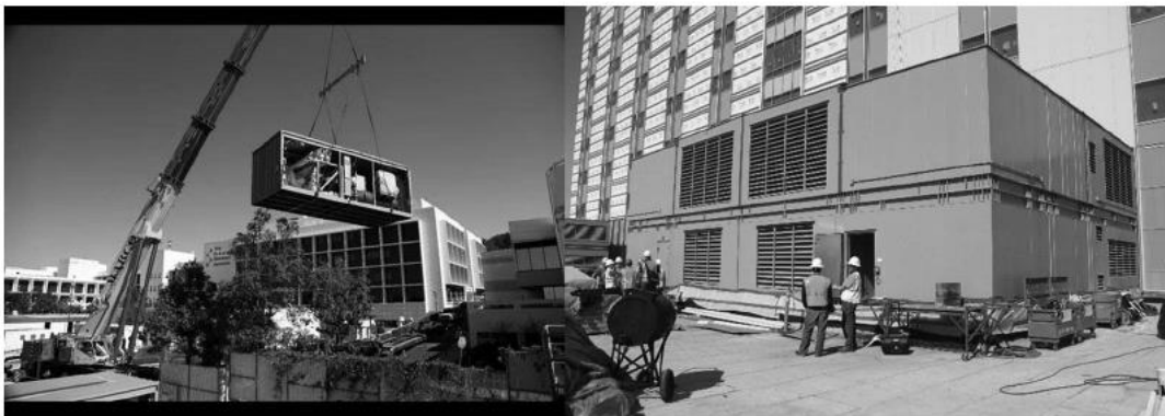
FIGURE C13.1-8 Premanufactured Modular Mechanical Systems
