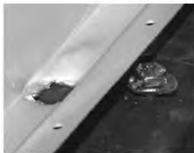
Failure of sheet metal base anchored with standard washer
